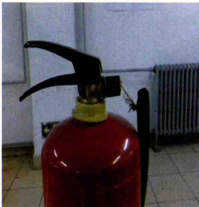
(a) 软管断裂
